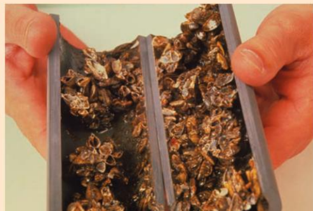
▲ Figure 6 A section through a water pipe which has been opened to reveal an interior clogged with zebra mussels, Dreissena polymorpha
